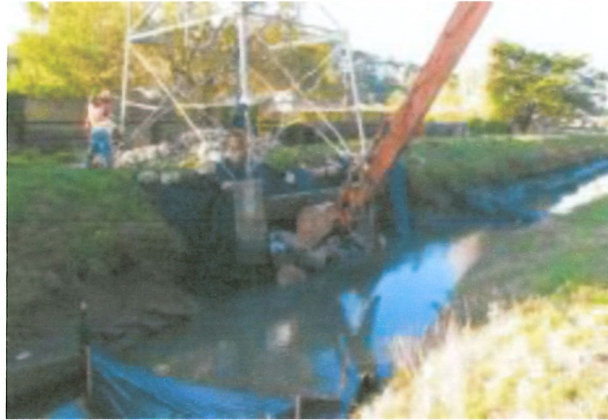
PG&E repair from storm damage in Tamalpais Valley. Credit Marin County DPW- page 328
